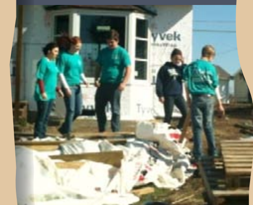
Catholic Charities workers and volunteers help to rebuild a house in Joplin.
