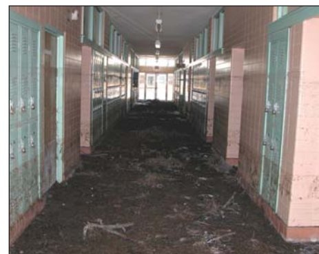
Dormitory Hallway, St. Stanislaus College Preparatory High School, Bay Saint Louis, MS.
